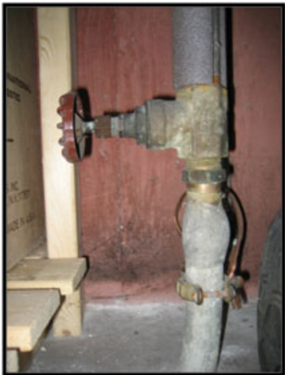
A Lead Service Line 39 Credit: EPA
